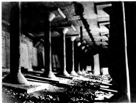
Photo 6. Joseph Jensen Filtration Plant, finished water reservoir. West wall at left, showing damage. Note failure at construction joint in roof and damaged columns. Metropolitan Water District photo.
